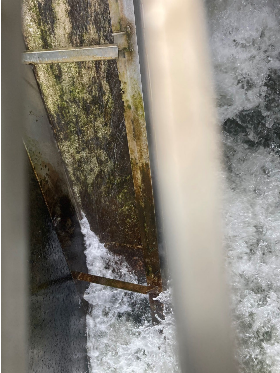
Broken angle iron on north entrance ramp of LPS with AWS flow surrounding ramp.
