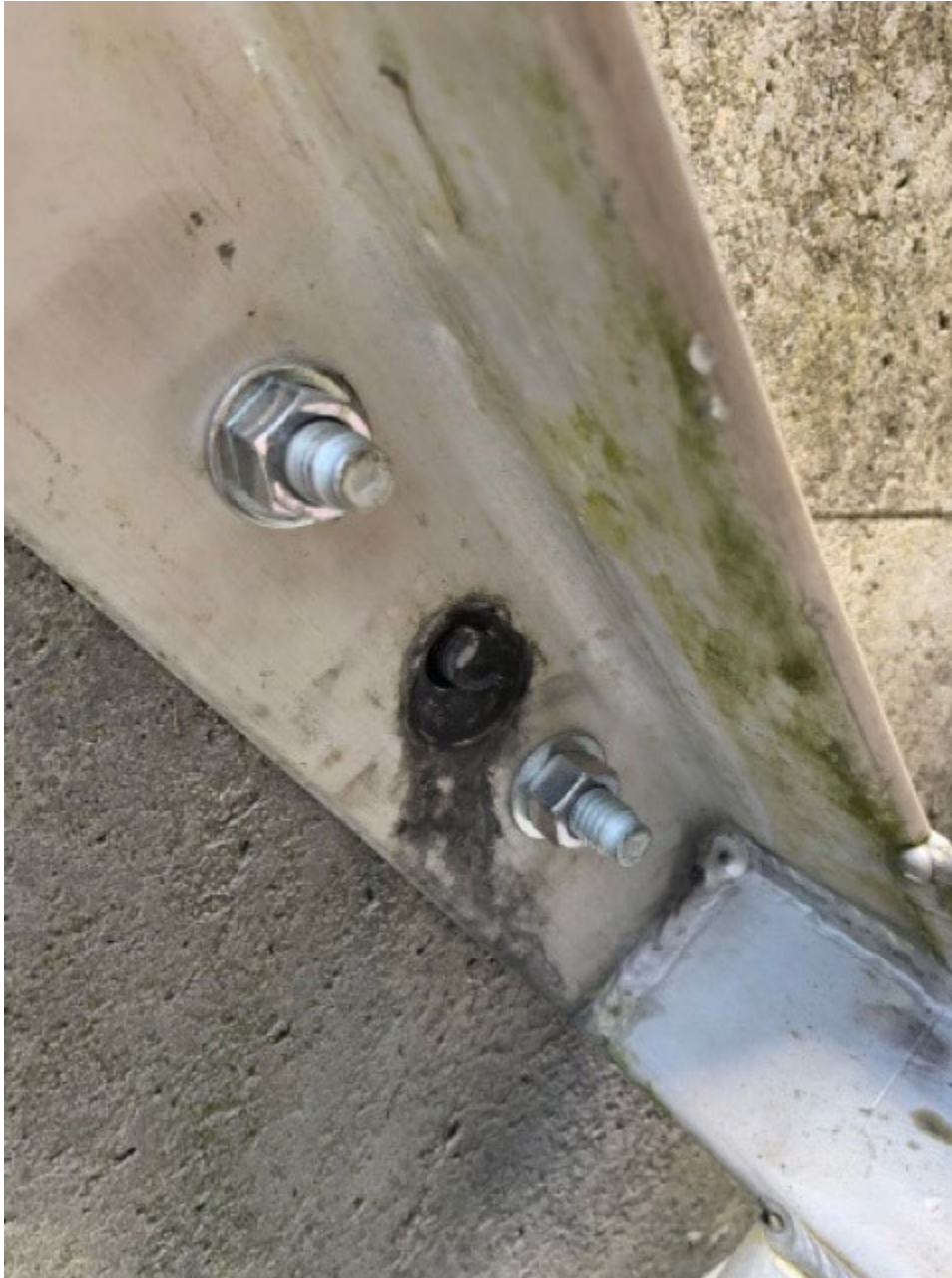
Sheared off bolt (middle) with two new bolts installed on 5/31 to help ramp stay in place until LPS dewatering
