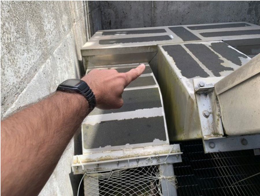
Crack at junction of rest box and north ramp.
