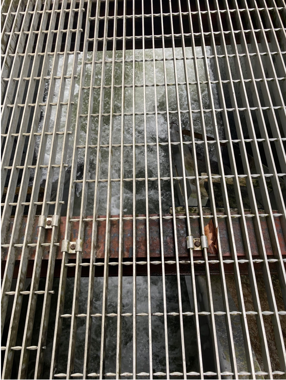
Photo looking downstream in AWS channel South ramp (left) and broken north ramp (right)
